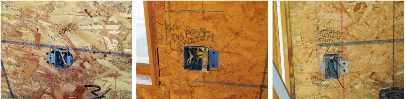
IMAGE 9.4 VARIOUS ELECTRICAL BOX INSTALLATIONS IN SIP WALLS
