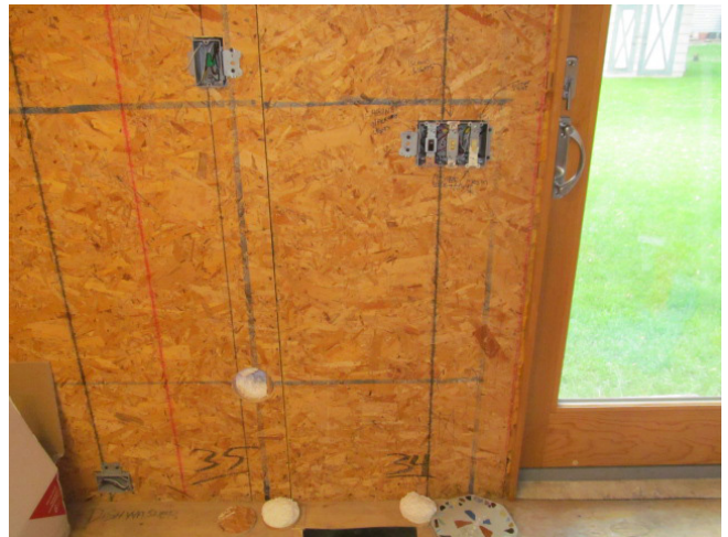
IMAGE 9.3 INSTALLED LIGHT SWITCHES AND OUTLET BOXES WITH OPEN ACCESS PLUGS NEAR DOOR.
